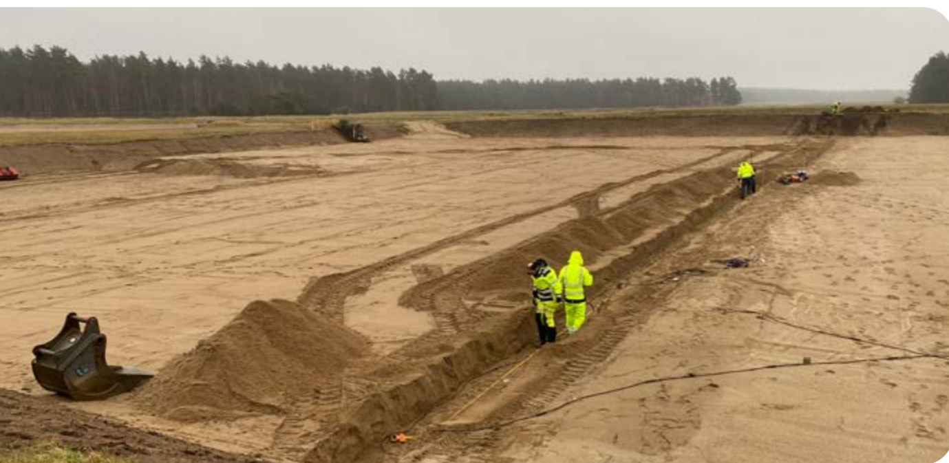
Installation of electrode spreads for geoelectrical monitoring intended to give an increased understanding of the processes below the water-filled infiltration pond. In the picture we see personnel from Engineering Geology, Lund University, deploying electrodes and cables in a trench that was backfilled afterwards.
